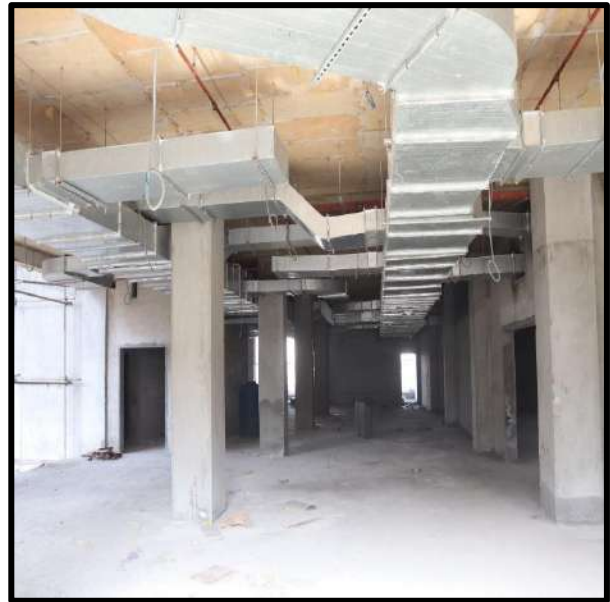
Picture 99: HVAC Ducting of PLGA Lahore
