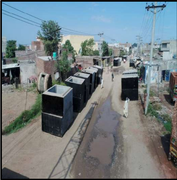
Picture 67: Single Cell Conduits laying is in progress near Sublime Chowk Site 1 Marala Road Sialkot
