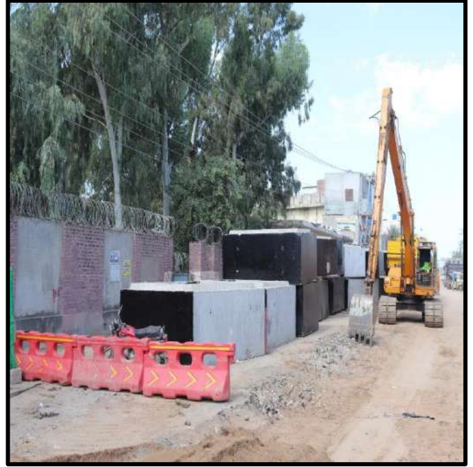
Picture 77: Conduits laying is in progress near Technical College Site 2 Marala Road Sialkot
