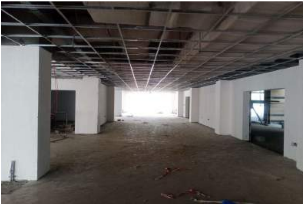
Picture 105: Inside View of PLGA
