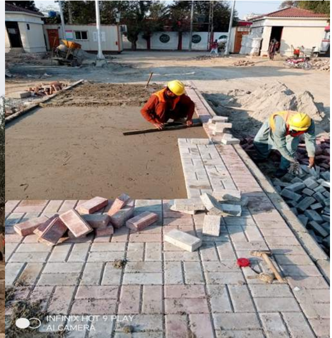
Picture 2: Laying of Tuff Paver on front walkway in Farid Town Park
