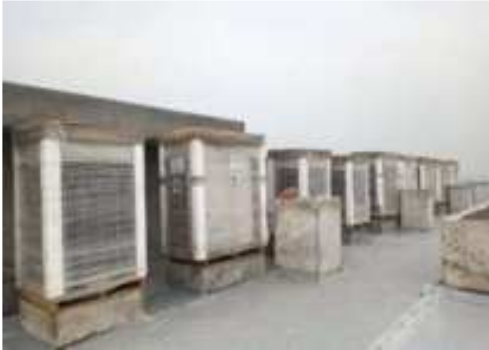
VRF system outdoor at roof top
