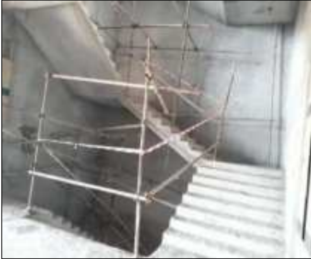
Hard railing and barrication on staircase
