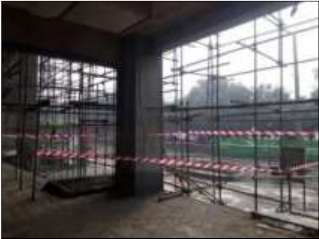
Use of barrication tape near edges at site
