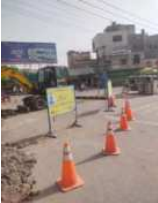
Sign board and Safety cones are placed on the Road for public awareness
