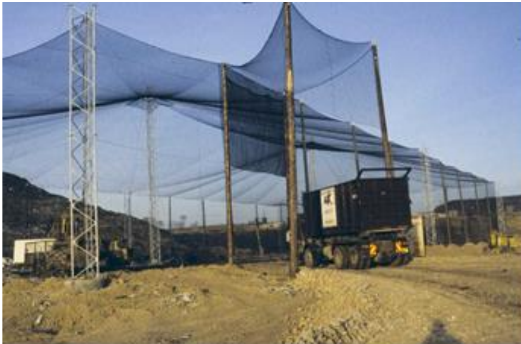
Figure 8-10: Example of a bird netting enclosure at an active tipping face on a landfill site
